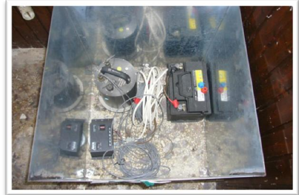
Photo 2: Inside of the BUT installation box
