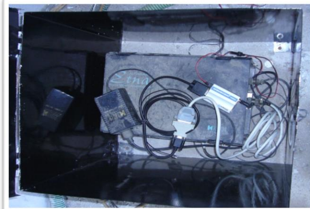
Photo 2: Inside of the E02 installation box
