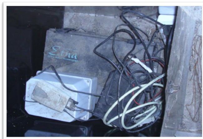
Photo 2: Inside of the E03 installation box
